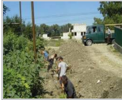
Works undertaken under the Drinking water supply systems in rural areas project, Moldova
